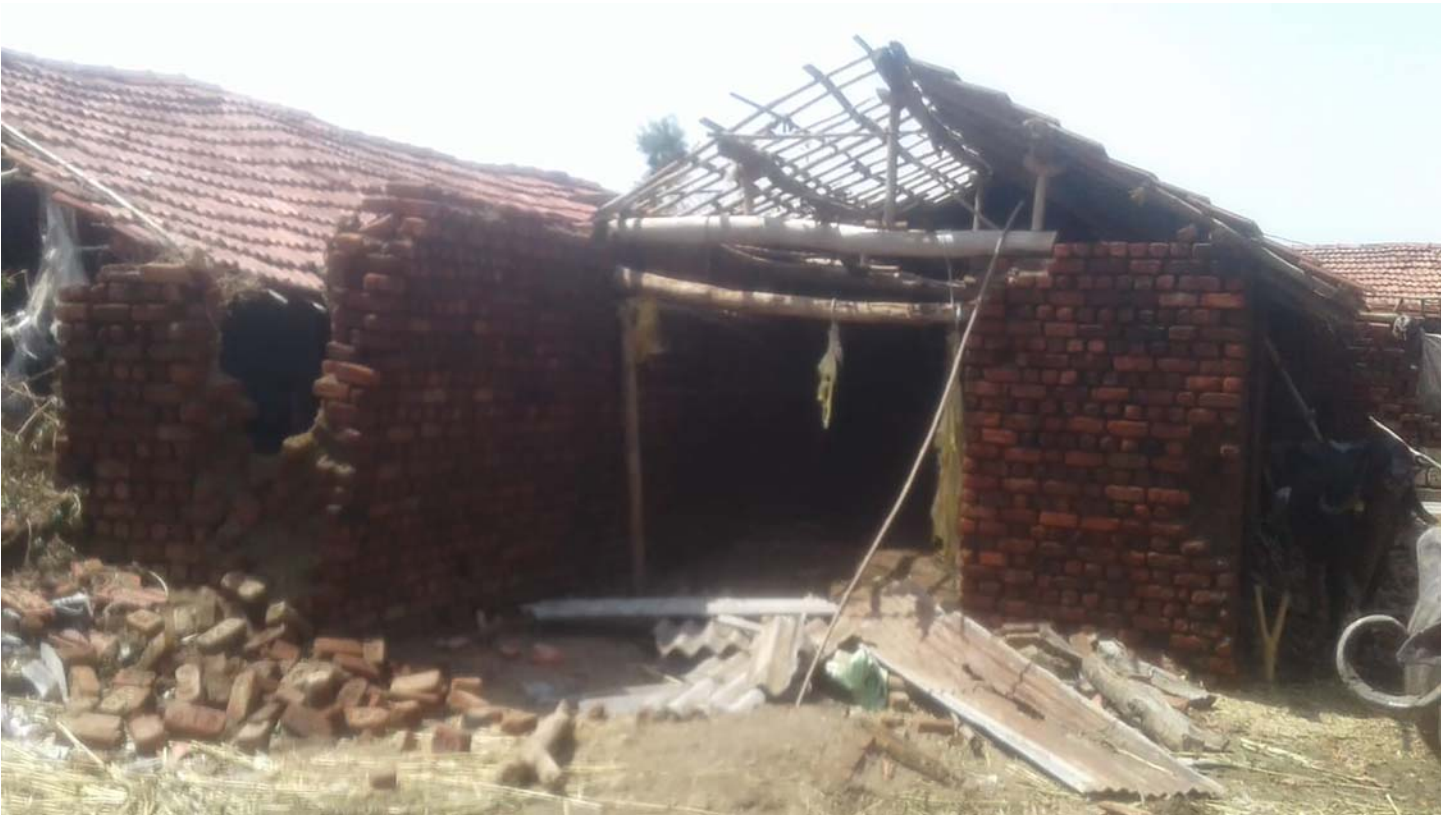
Cyclone destroyed believer's house in Gujarat
