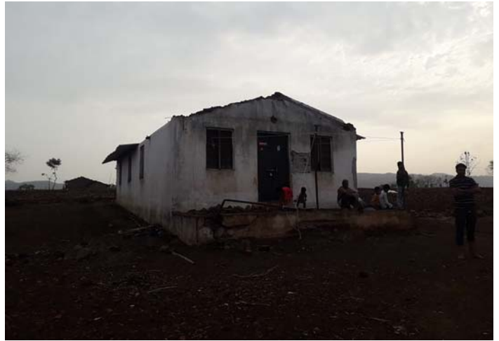
Ps. Bhursing's ANLMC Church roof collapsed in Badwani, MP due to heavy rain
